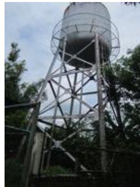
Figure 5: Community water tank
