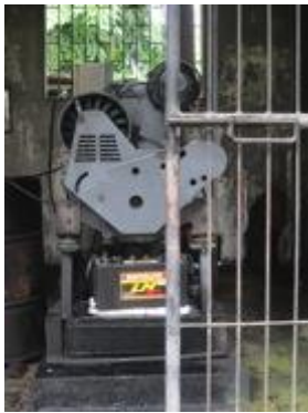
Figure 4: TG-09 deep well pump
