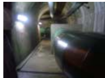
The pipeline at the Casecnan Project
