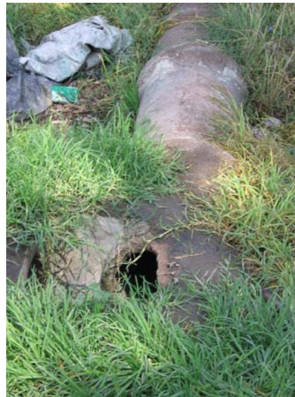
Irrigation system in Zumpango
